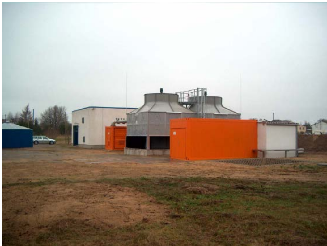
Figuur 4.3: Neustadt-Glewe Geothermal Heating and Power Plant
