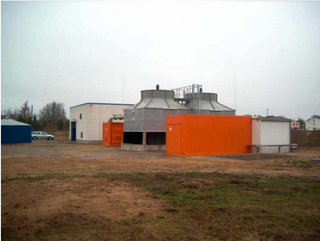
Figuur 4.3: Neustadt-Glewe Geothermal Heating and Power Plant
